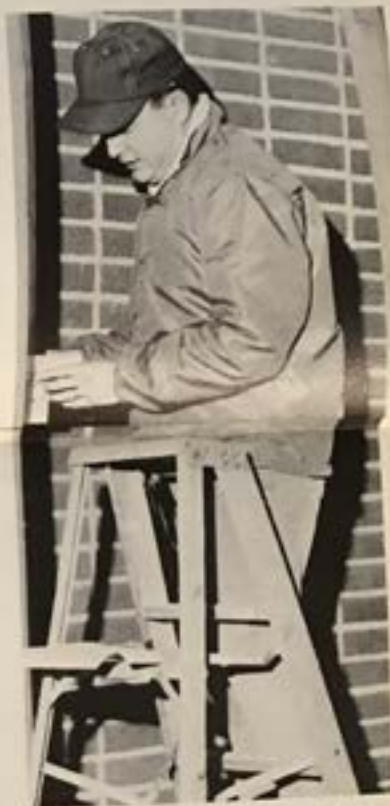
He donated his Christmas vacation time to build a new training room.
