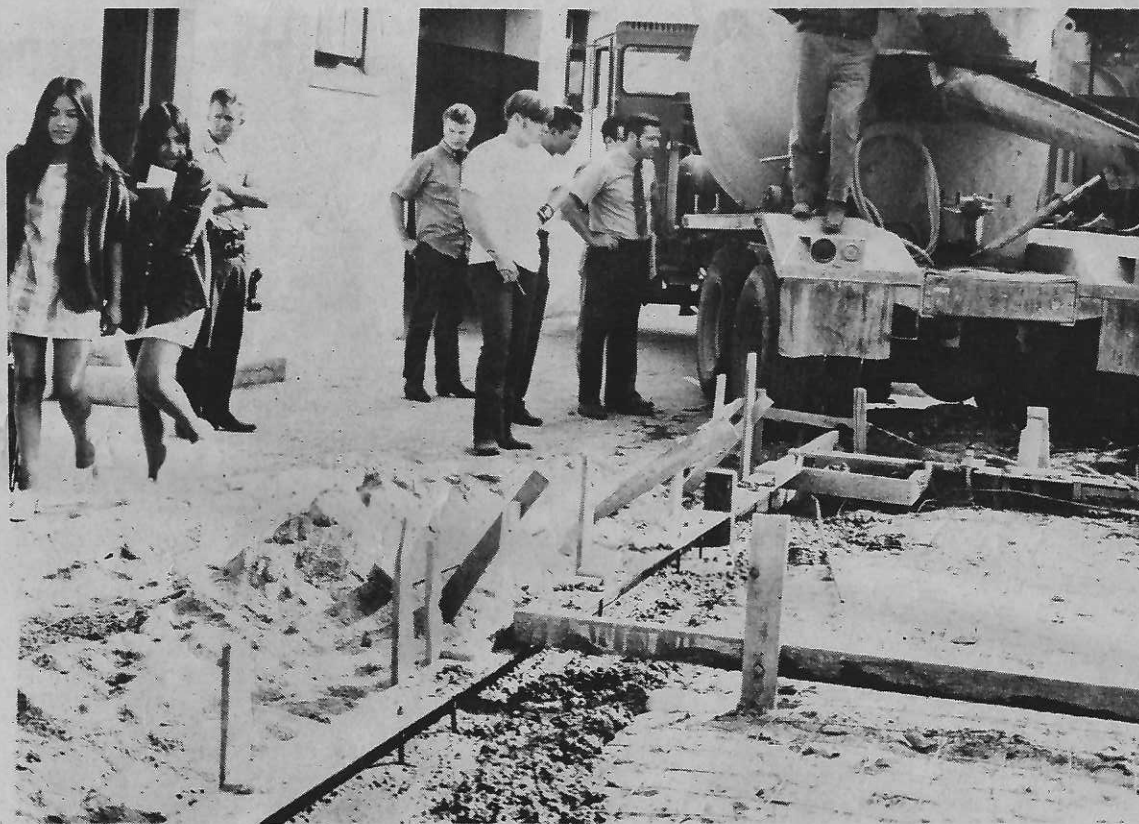
PASSING BETWEEN CLASSES students stop to watch the construction of the new crafts building while. Mr. Larry Anderson tries to help supervise. The building is to be finished by Nov. 13.
